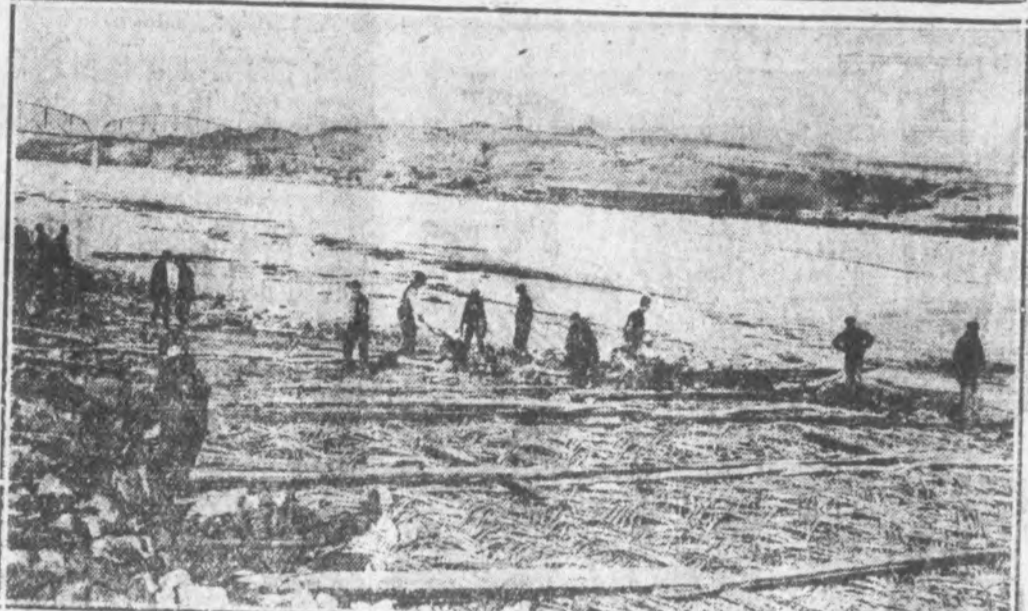
Workmen are shown rushing the work of riprapping the banks of the Missouri River, near Medan, N. D., in fear of Spring floods. Willow mats, weighted with rock, are used to protect the land from the swollen stream.
