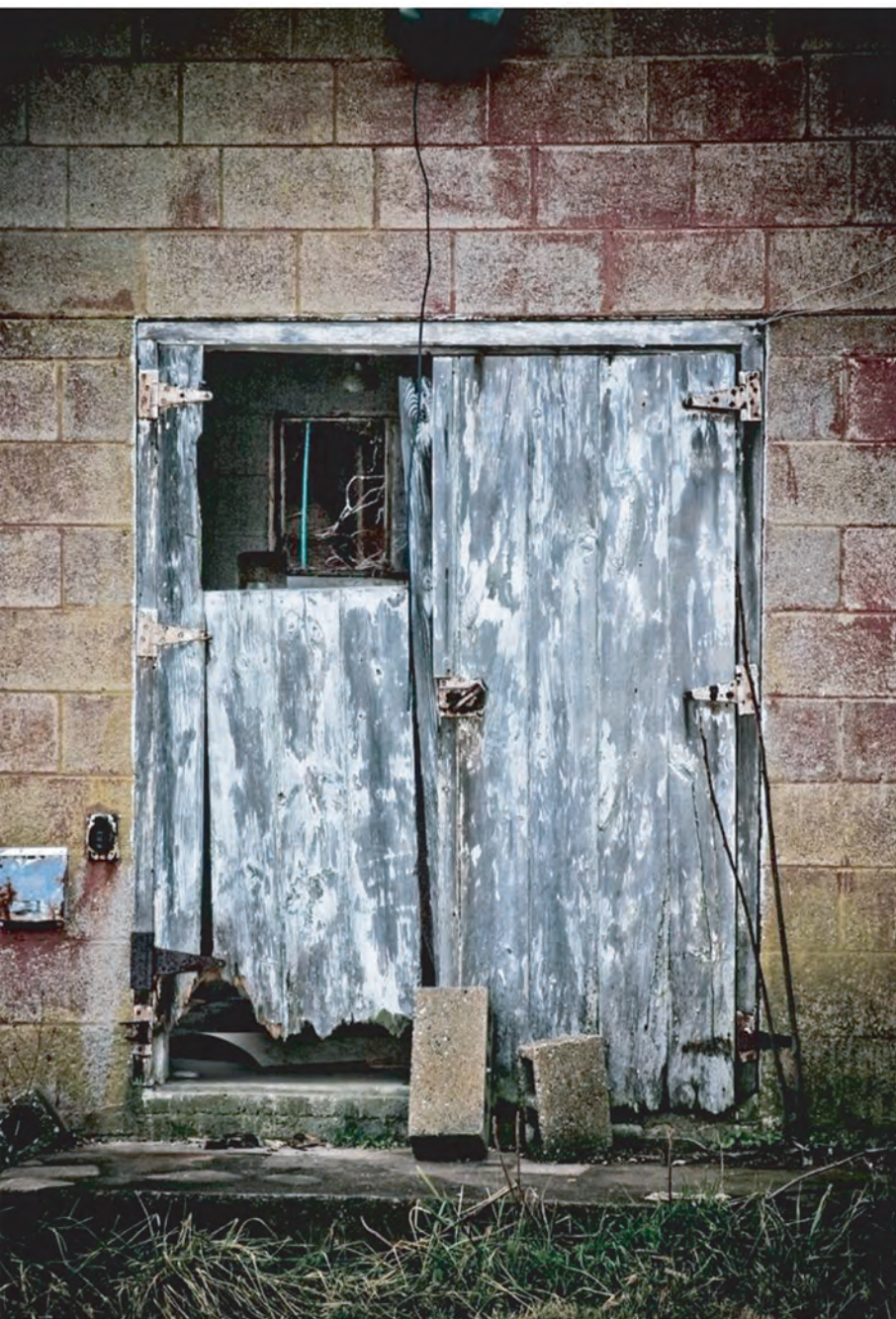
Broken Doors - Gregory Harris, MS2 - Photography
