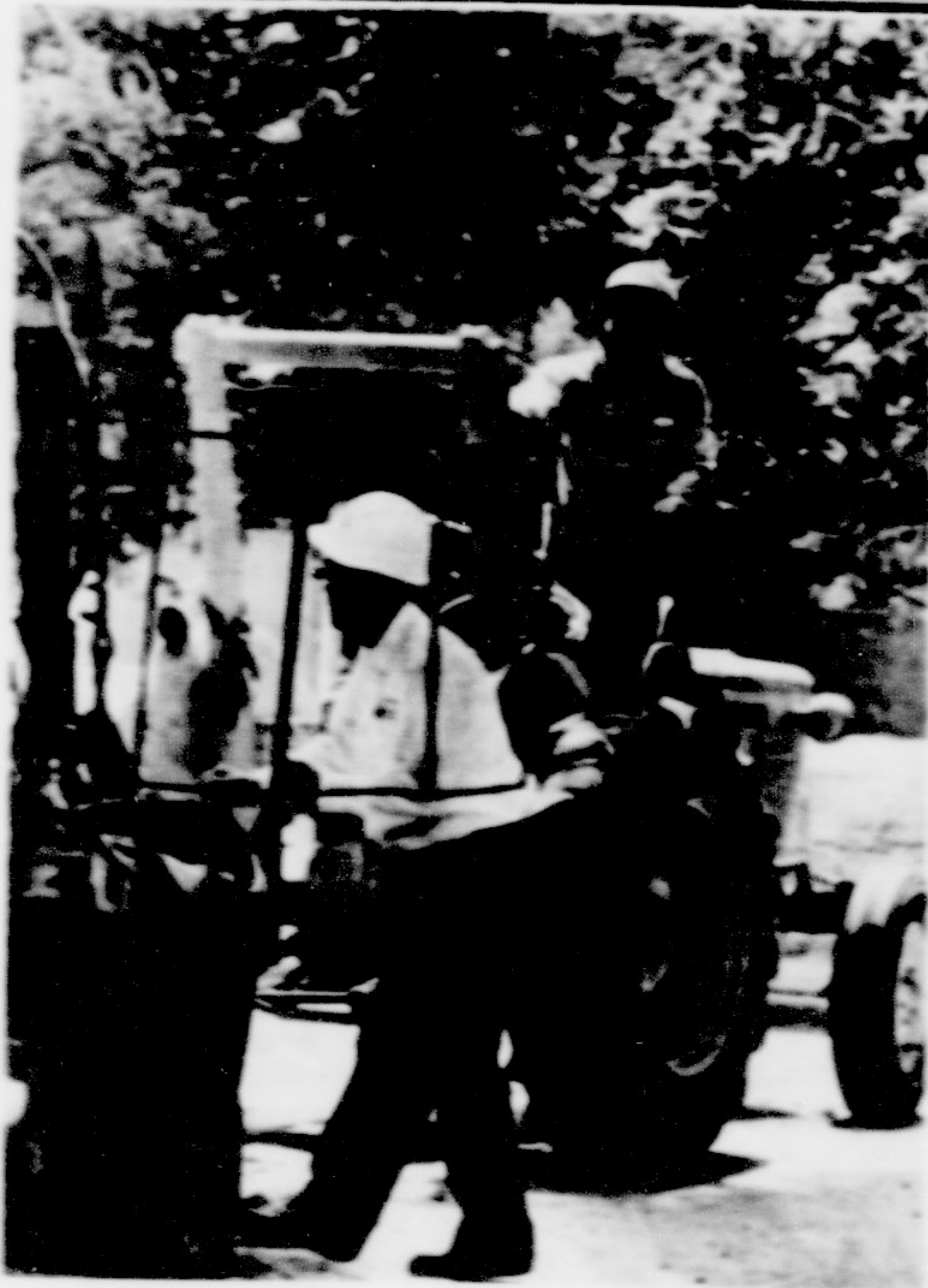
Maintenance crews have been working hard making necessary repairs on campus sidewalks.
