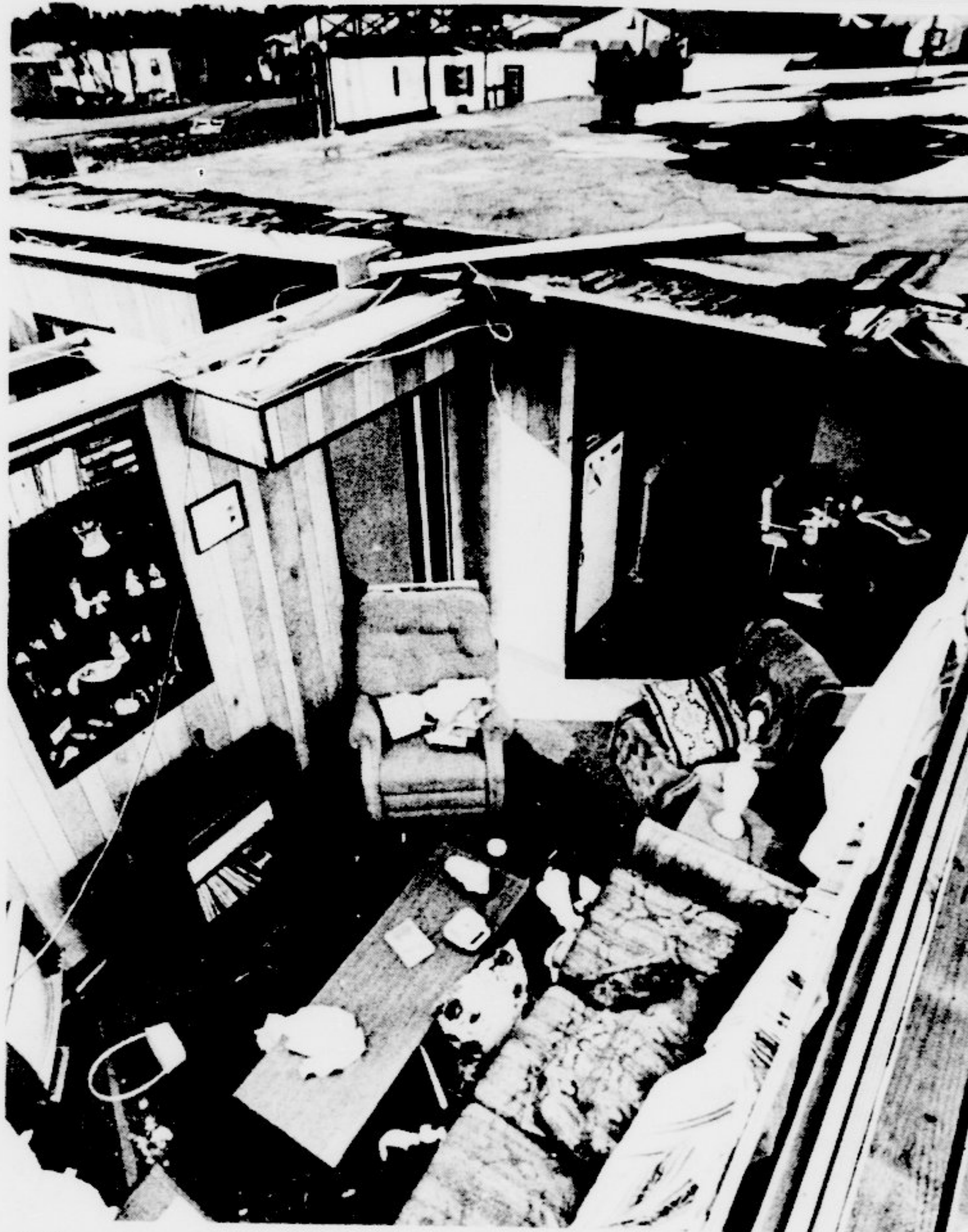
When the roof of a house is missing, an interesting view can be obtained from above. This house at Carolina Beach was damaged by Hurricane Diana.
