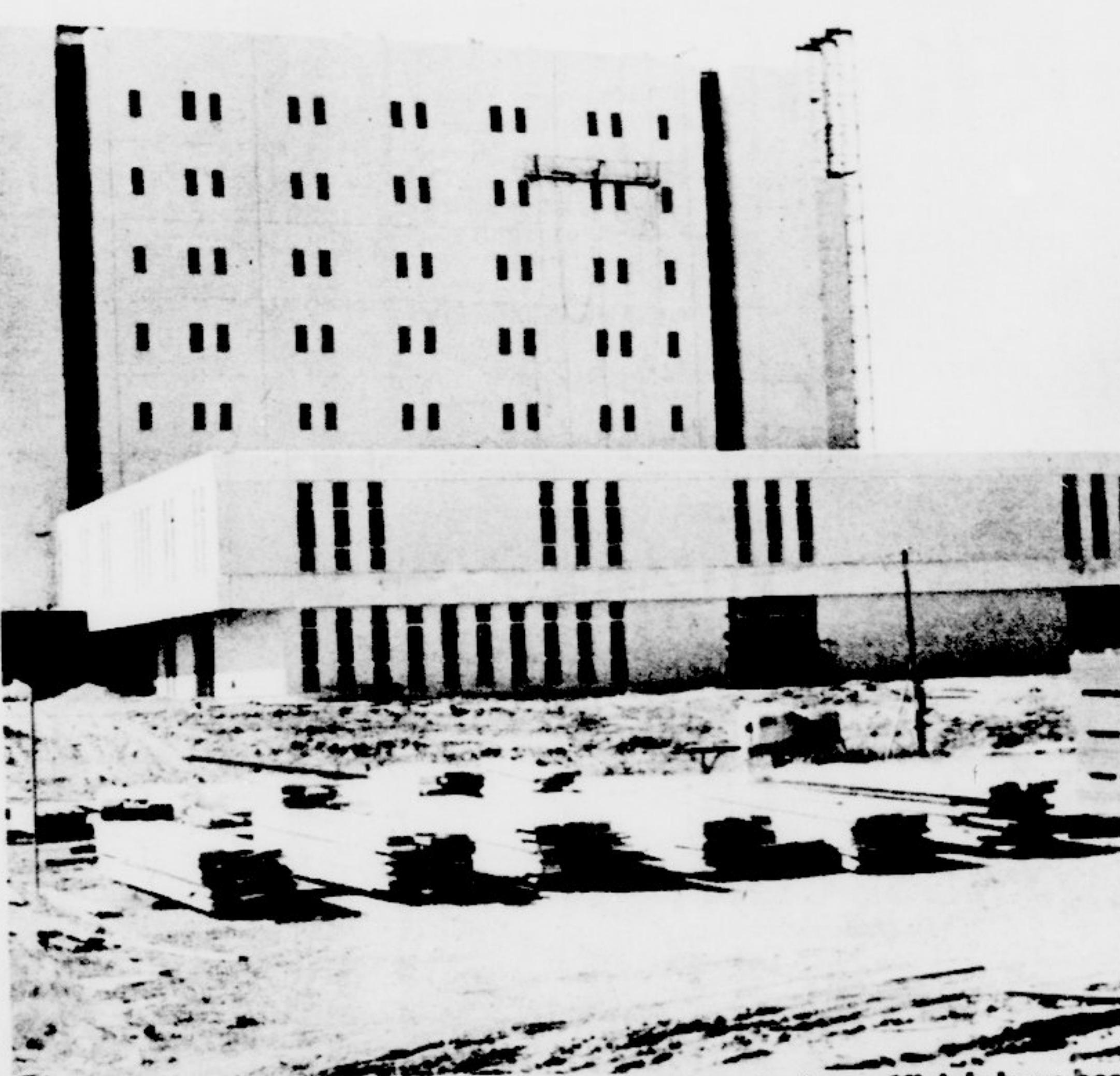
Despite the conspiracy indictments involving bid rigging, officials have been assured that work on the medical school complex will continue.
