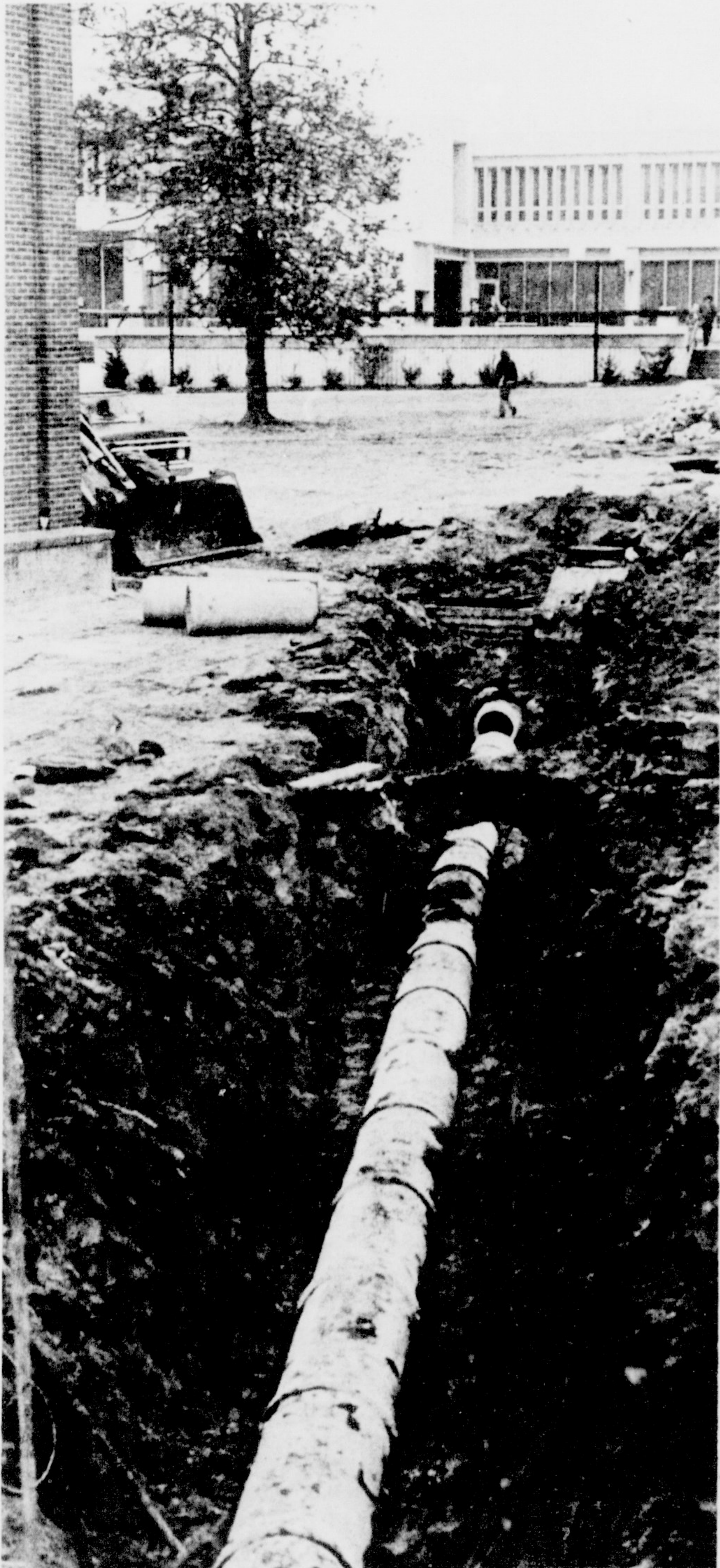
ECU's VERSION OF the Alaskan Pipeline will carry drainage water in the low lying area between Joyner and Mendenhall.
