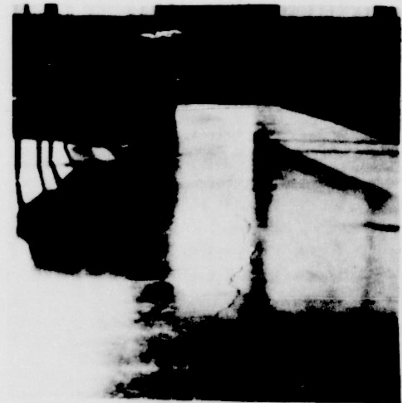
CRACKS APPEAR SHORTLY after construction.
