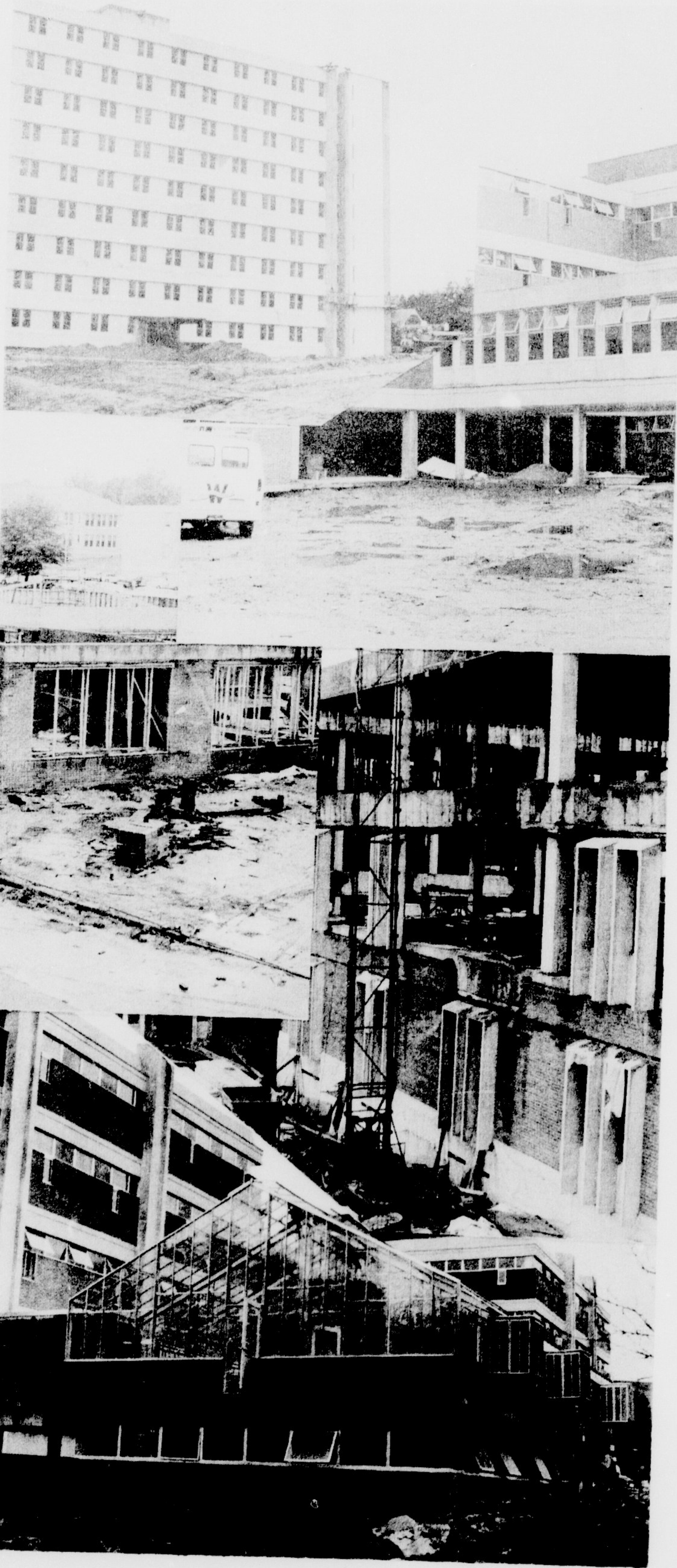
Pile drivers have given way to steel beams and thick cables on the eastern end of campus, as East Carolina continues to build its physical plant.
