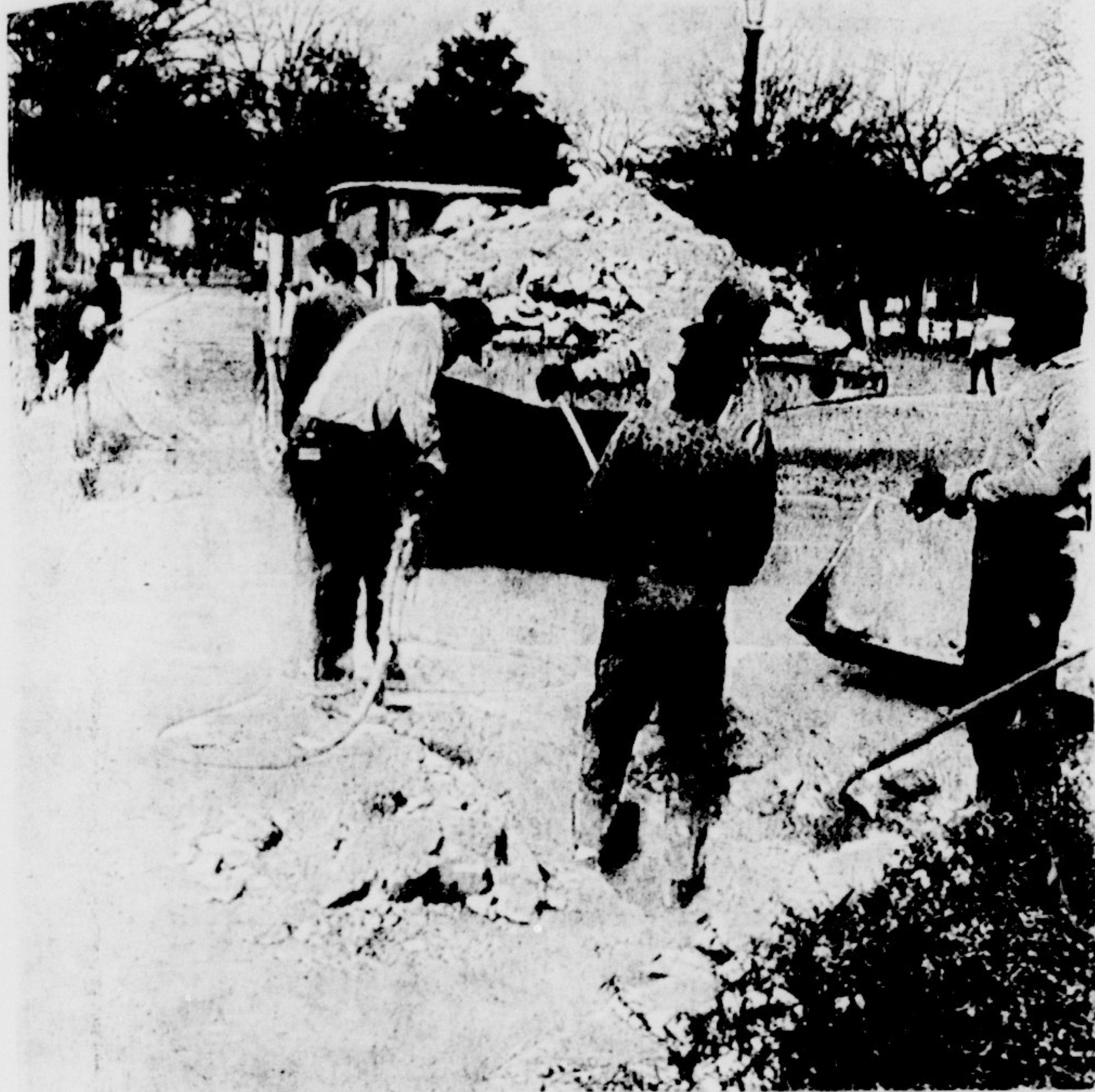
MECHANICAL MOLE —Do you dig the East Carolina campus? Evidently someone does. Utility men are in the process of replacing all of the campus underground wires with new cables.
