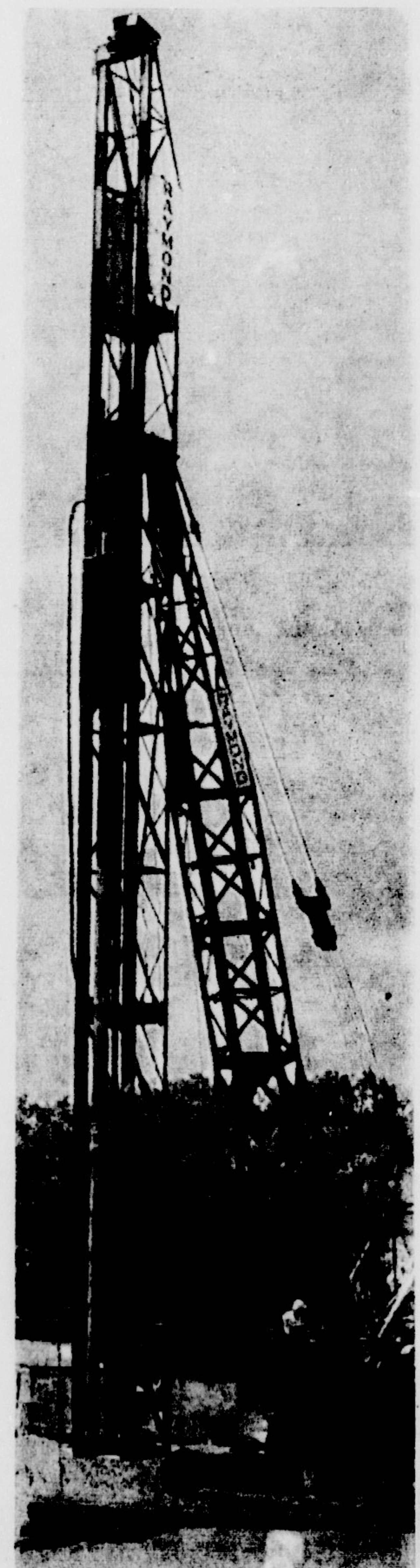
RAYMOND —Raymond, despite his noise and tendency to disrupt classes, is making a worthwhile contribution to East Carolina University, as he drives the pilings for the construction of new classroom buildings. (Photo by Quade)
