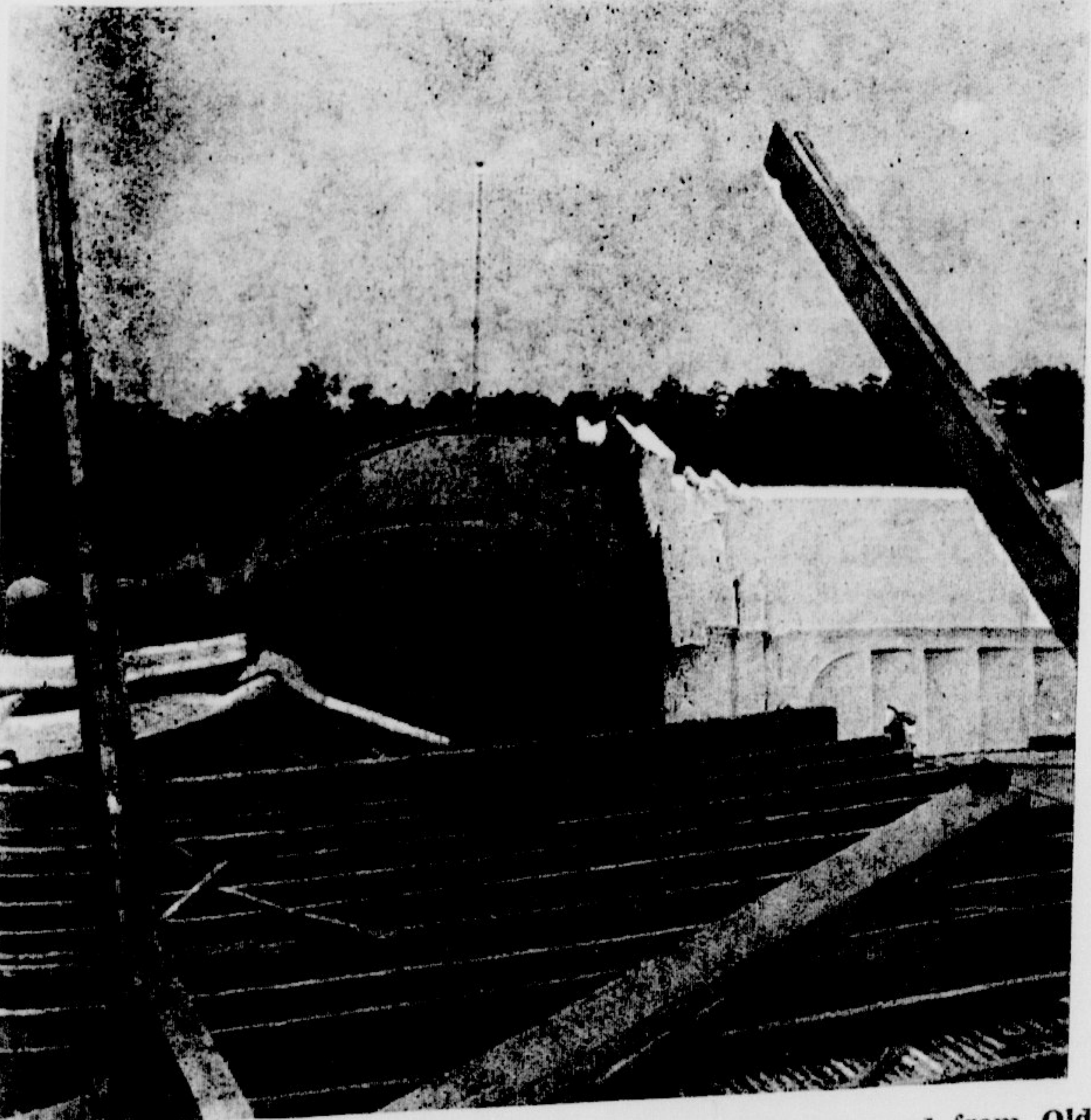
AFTER FALL — The Bell Tower was never safely removed from Old Austin; it fell Tuesday morning, when the movement of a demolition bulldozer caused the building to vibrate and the dome-like structure to fall.
