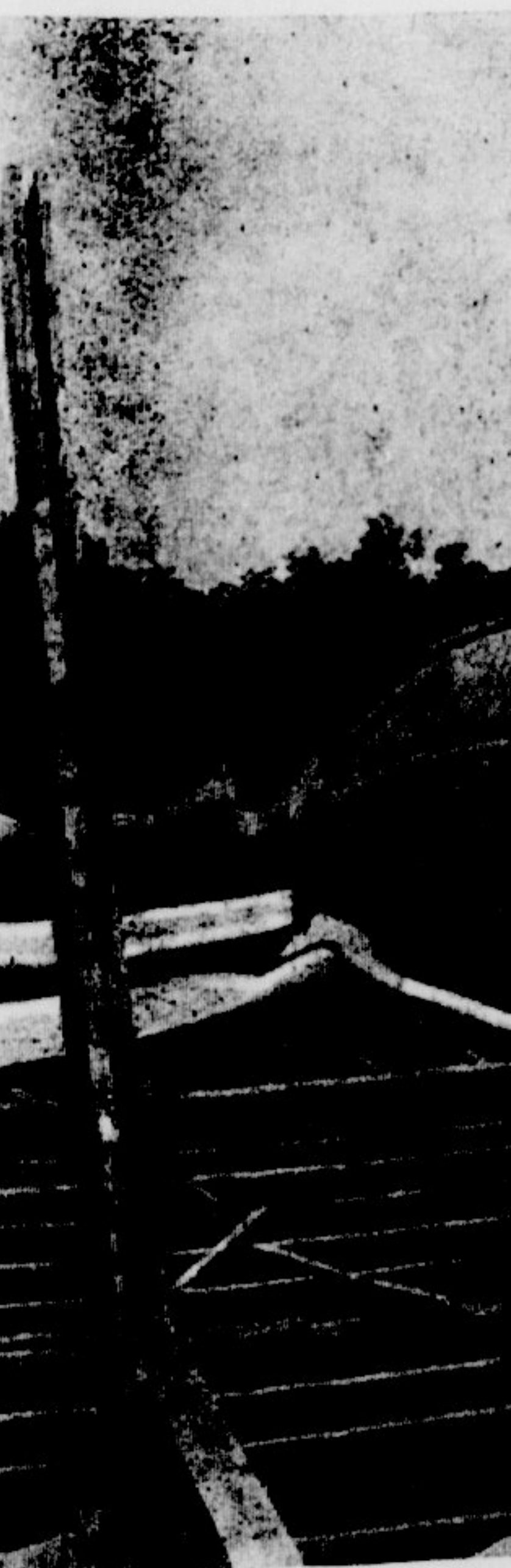
AFTER FALL — The Bell Austin; it fell Tuesday m bulldozer caused the buildi fall.
