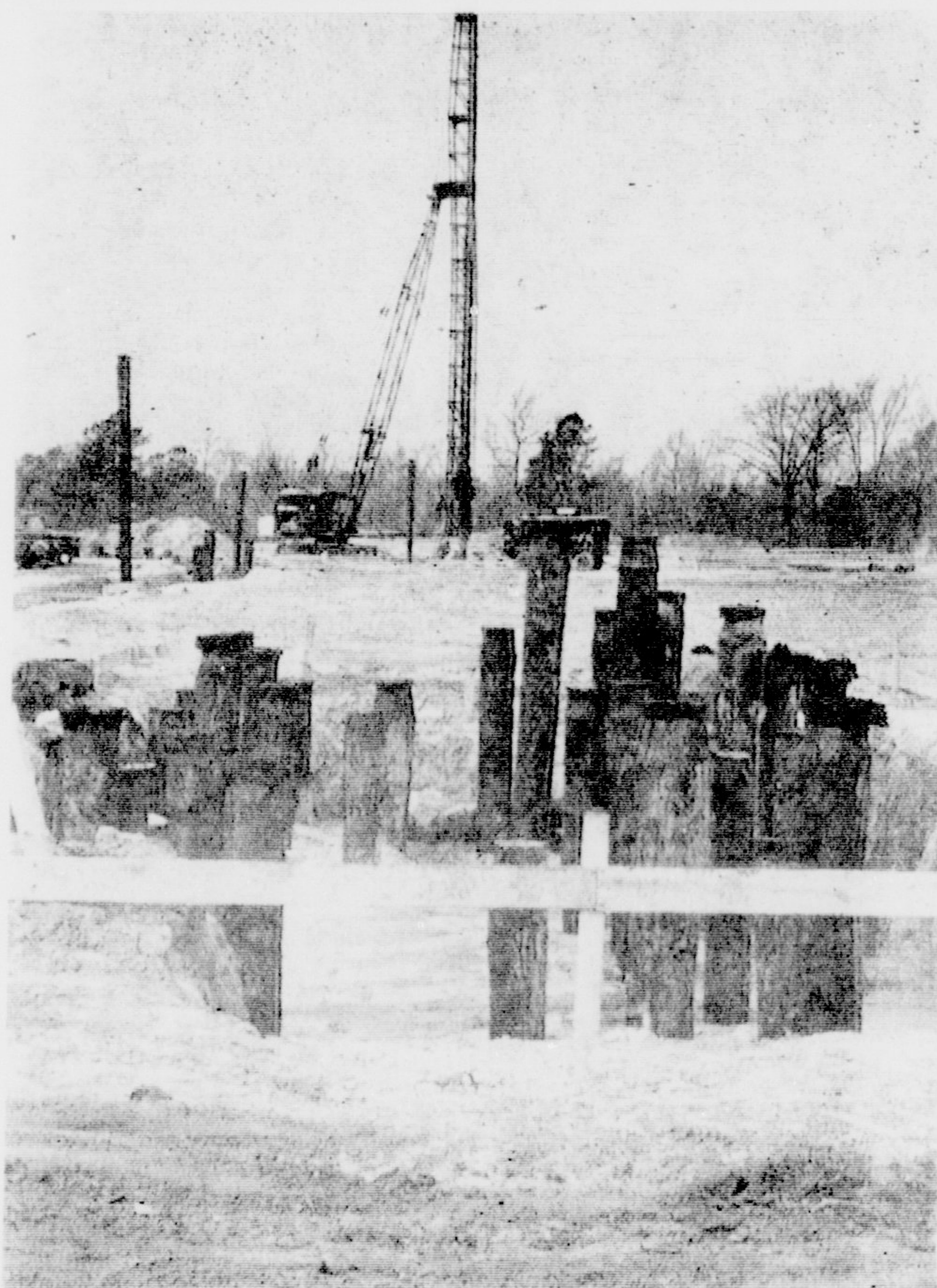
Construction is well underway for the new coliseum which is planned for completion sometime next year ('68).
