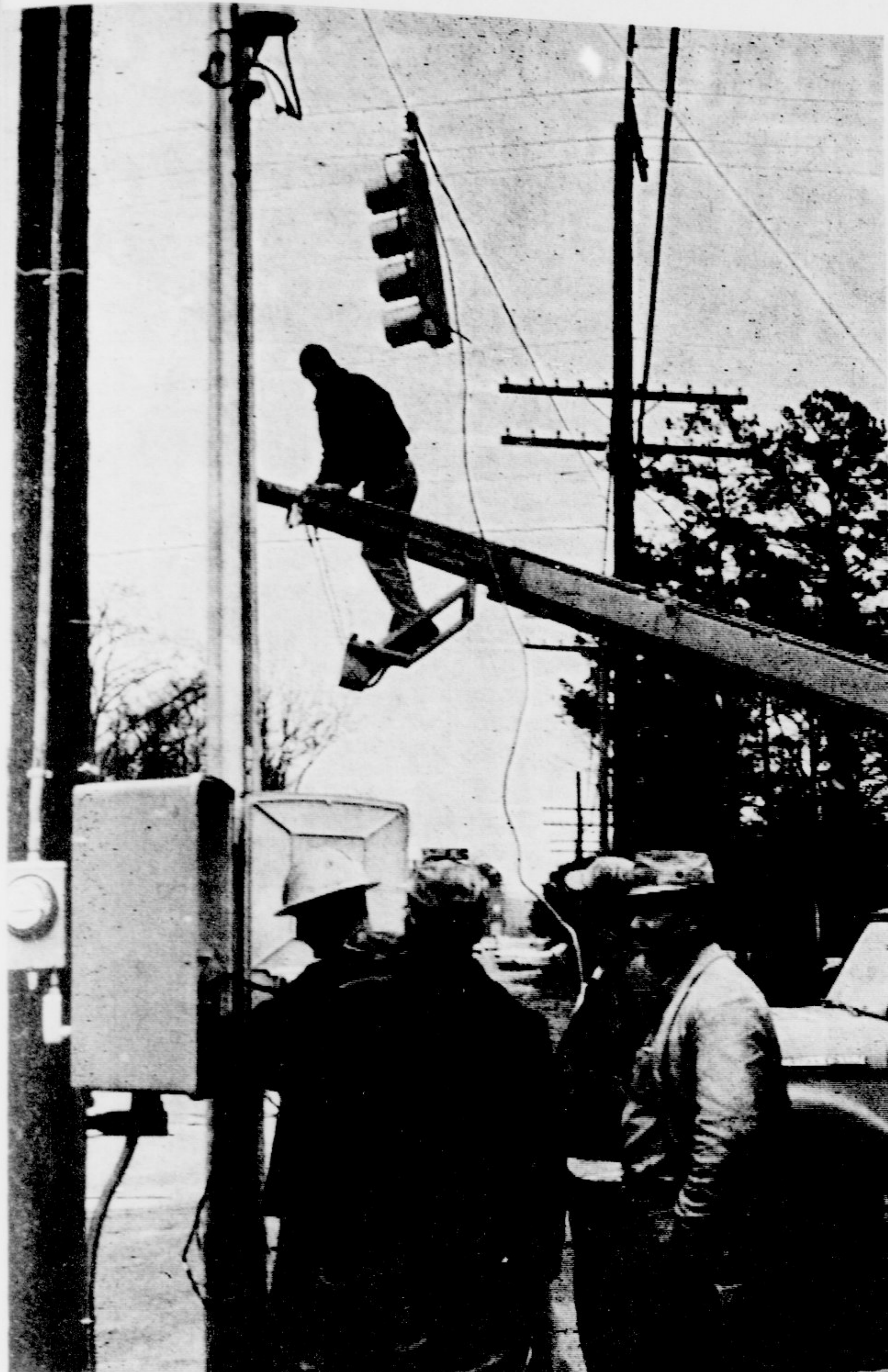
WUAHOO! At last we have that long hoped-for stop light on Tenth Street. What's more, we even have our own special control signal box! Here the State Highway Commission installs the stop light and checks it out to be sure that operations are to full capacity.
