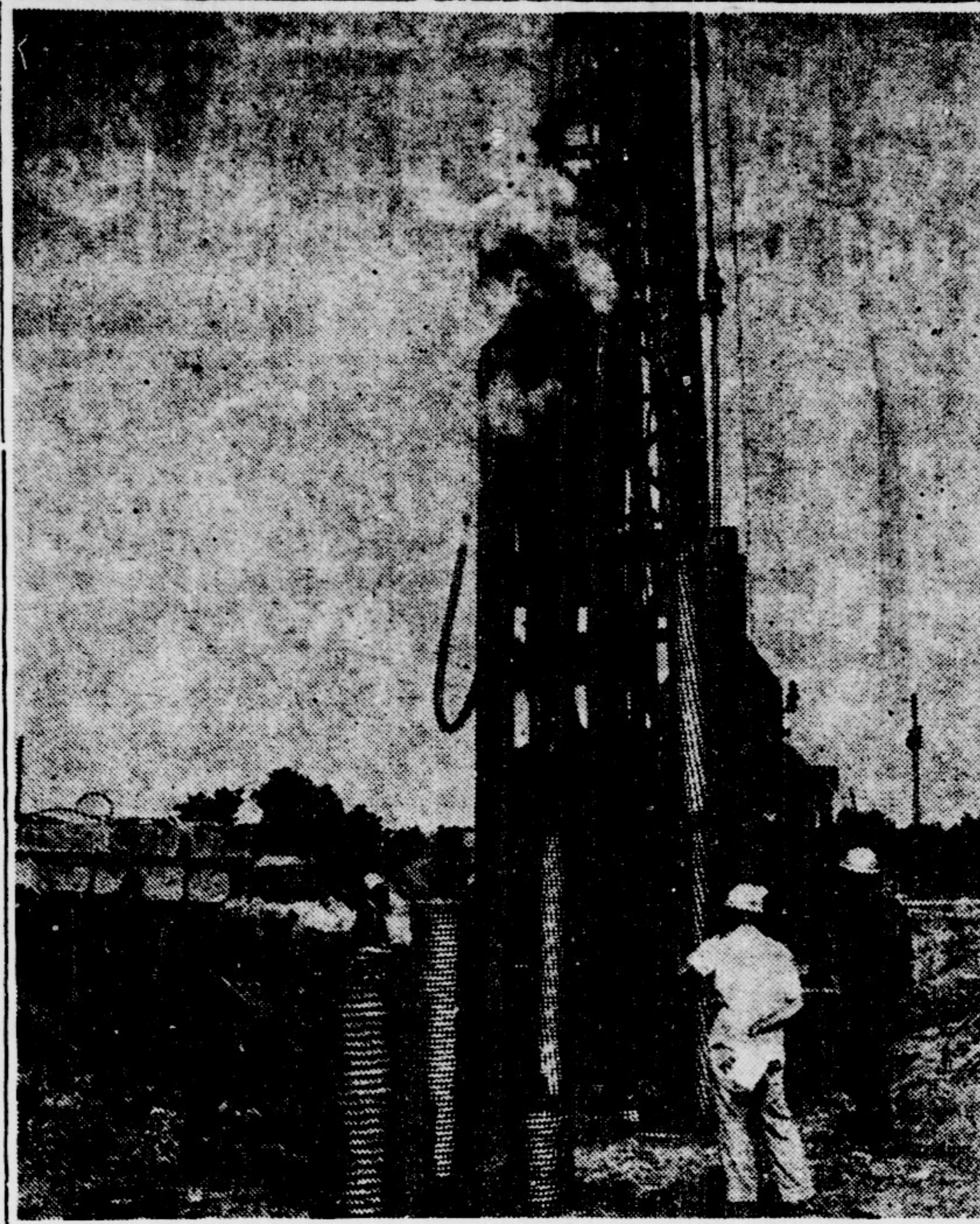
CONSTRUCTION CONTINUES . . . on EC's expanding campus. Above is the beginning of another men's dormitory, one of several that will spring up in the near future. —Photo by Jim Kirkland
