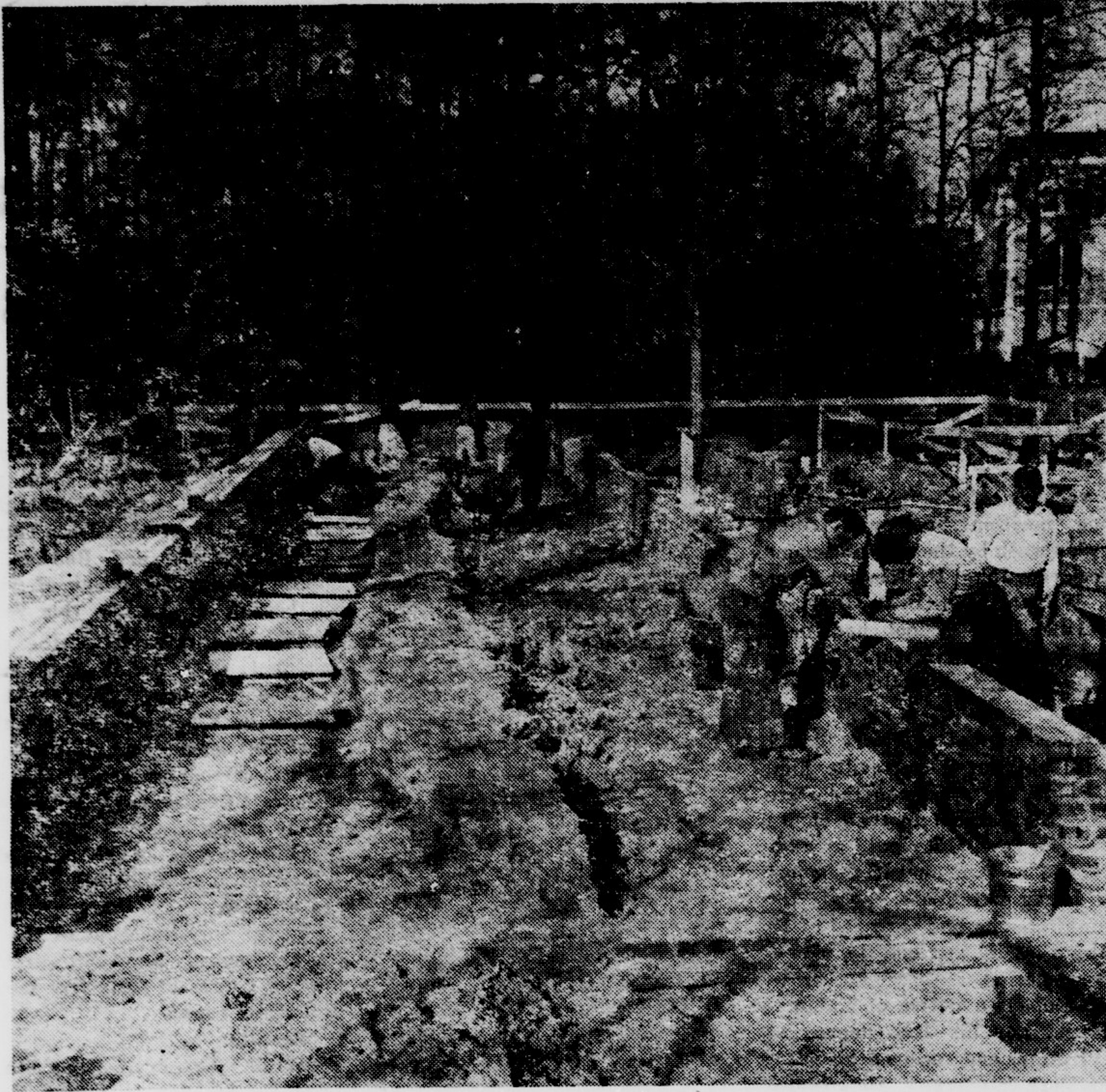
Above is a picture of the work on the foundation of Slay hall, the new men's dormitory on the campus. The building, which will be a brick construction with limestone corners, will house around 216 men and will probably be completed sometime late this fall.
