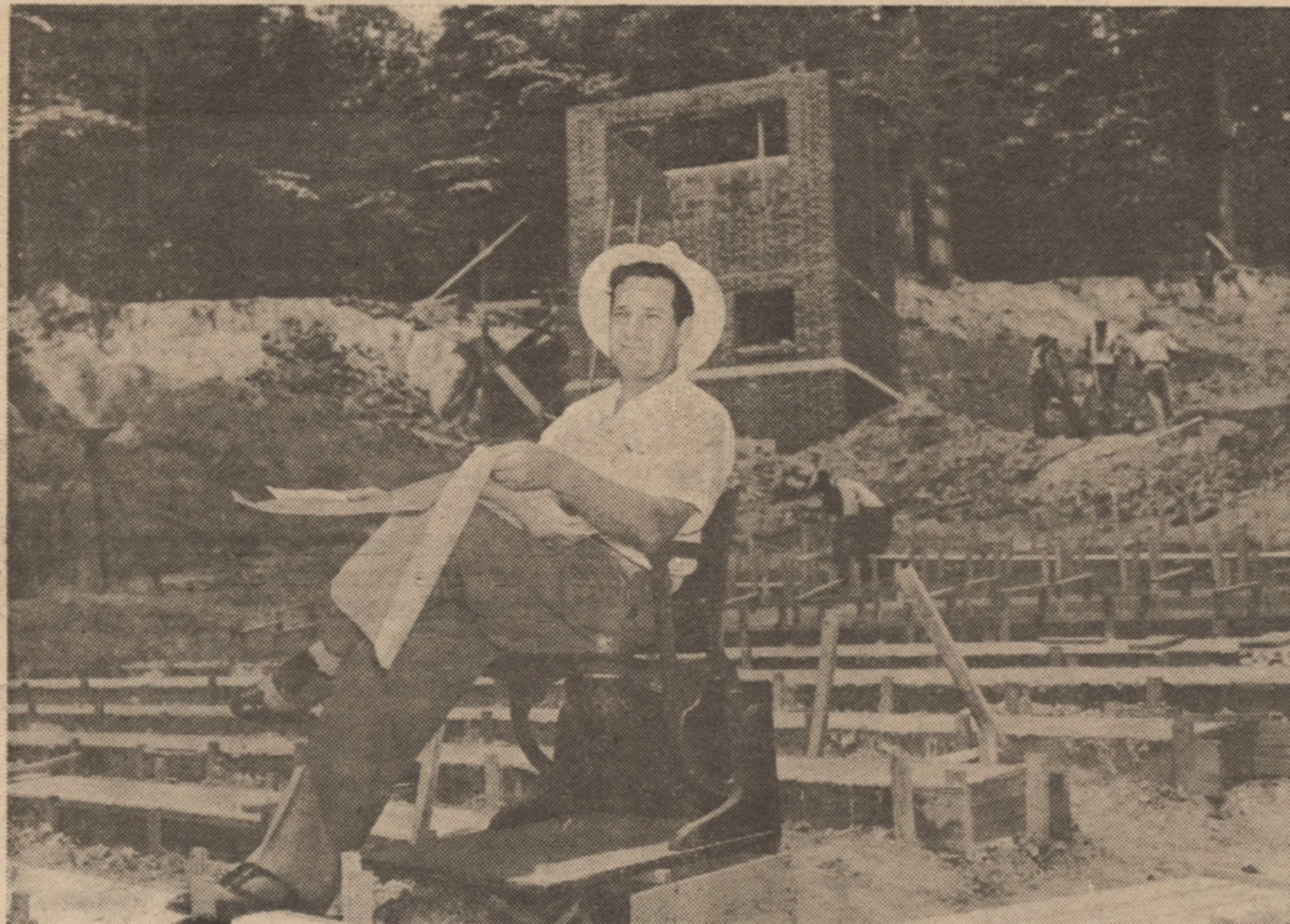
Green does some "sidewalk superintending" as the amphitheater begins to take shape around him.
