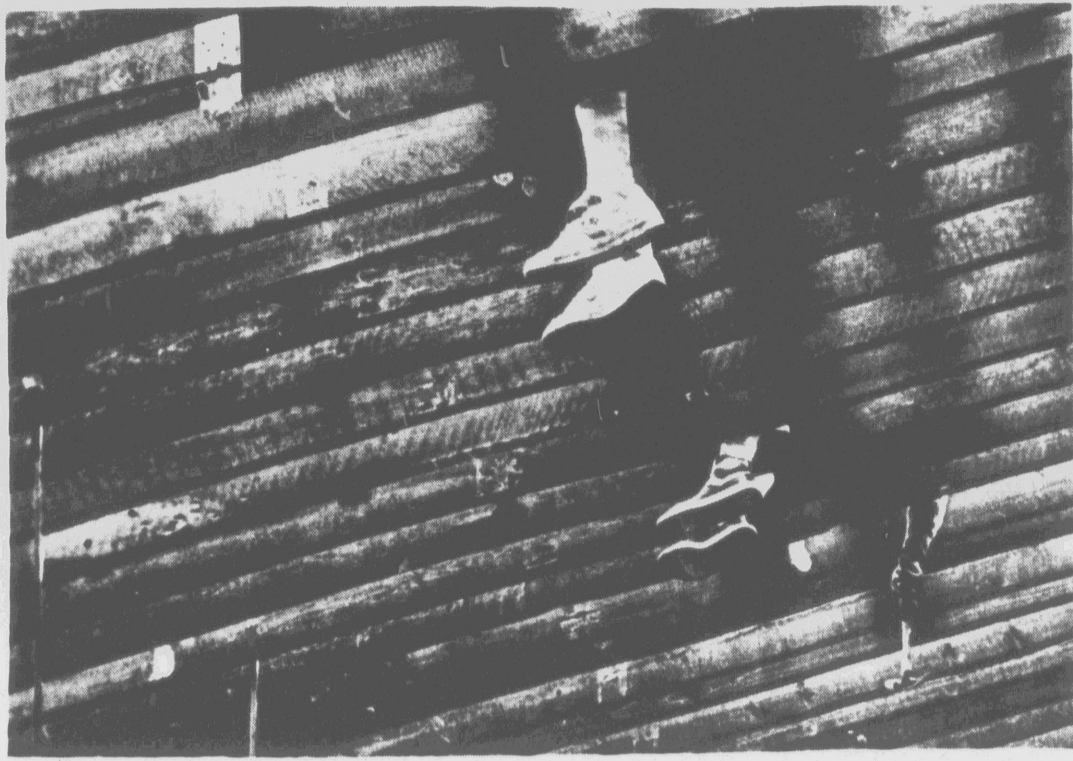
HANGING FEET — Workers dismantling an old warehouse recently on the Tar River near Tarboro let their feet hang through the rafters while they worked. (AP Laserphoto)
