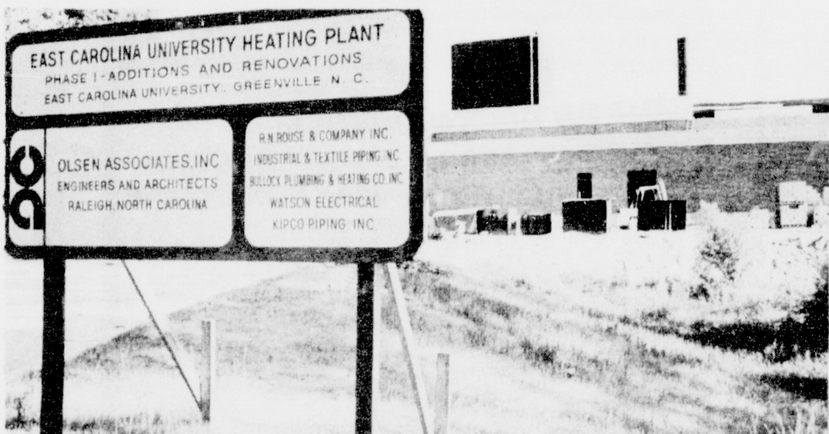
NEW ECU HEATING PLANT--The new ECU heating plant is located on 14th St. and is scheduled for opening soon. The fuel oil system will take the place of the coal burning system on campus.
