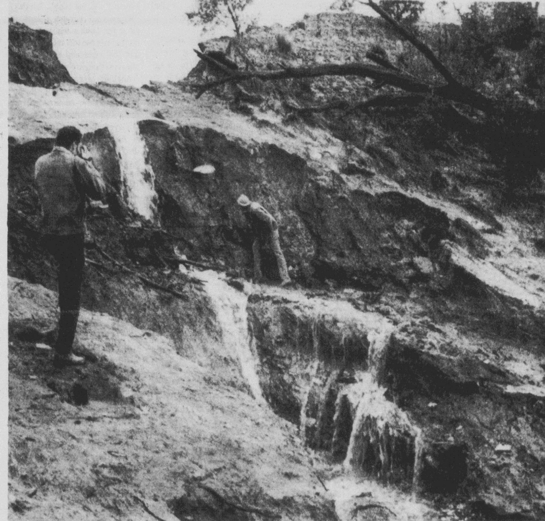
WHERE DAM BROKE — An engineer with the Department of Natural and Economic Resources photographed the remains of an earthen dam that
