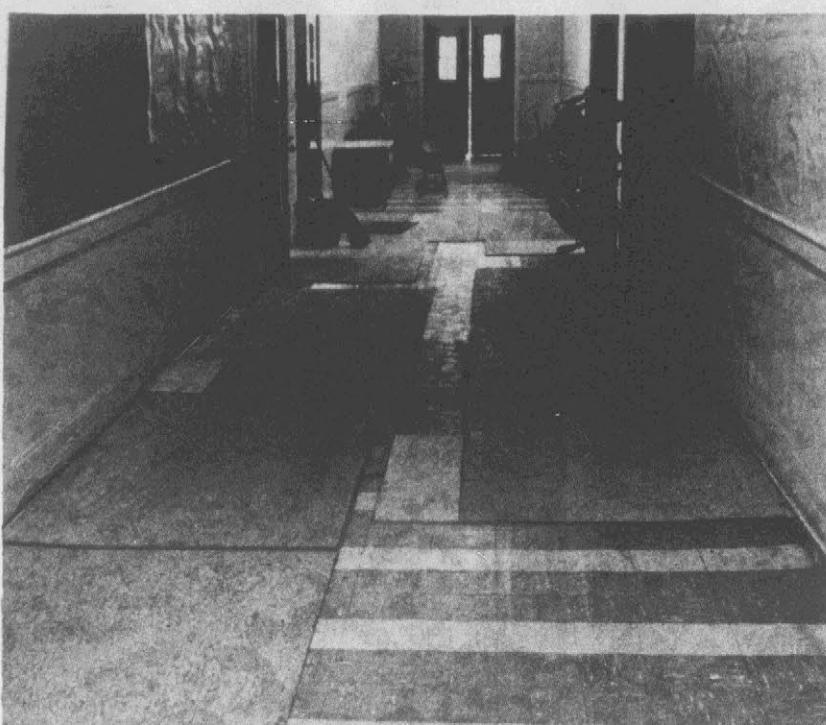
PLYWOOD ... covers weak and rotted sections of flooring at Third Street School. This school, condemned shortly before the end of the 1975-76
